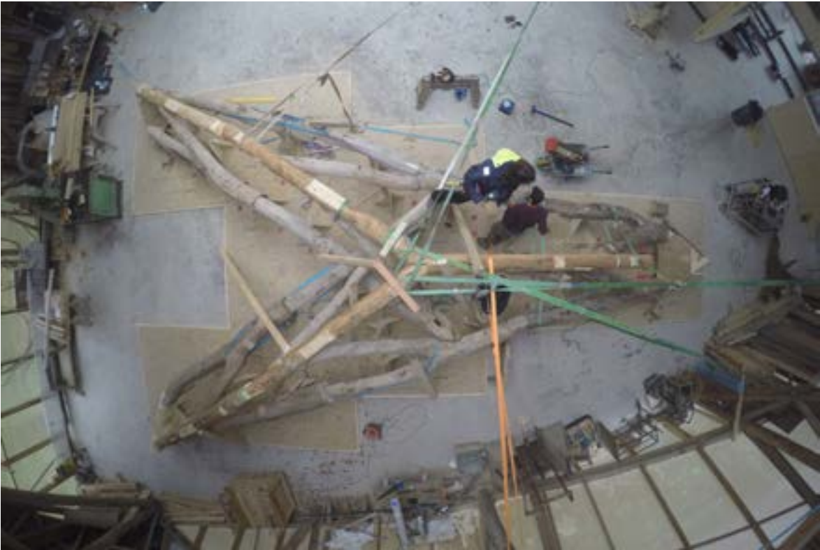
Fig. 22. Designed and fabricated with digital precision, a number of forks required some encouragement to align properly. Here, points are tied back to the structure of the Big Shed with ratchet straps.
