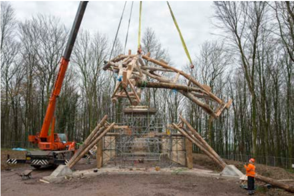
Fig. 24. Front half of the Tree Fork Truss being craned in to position.
