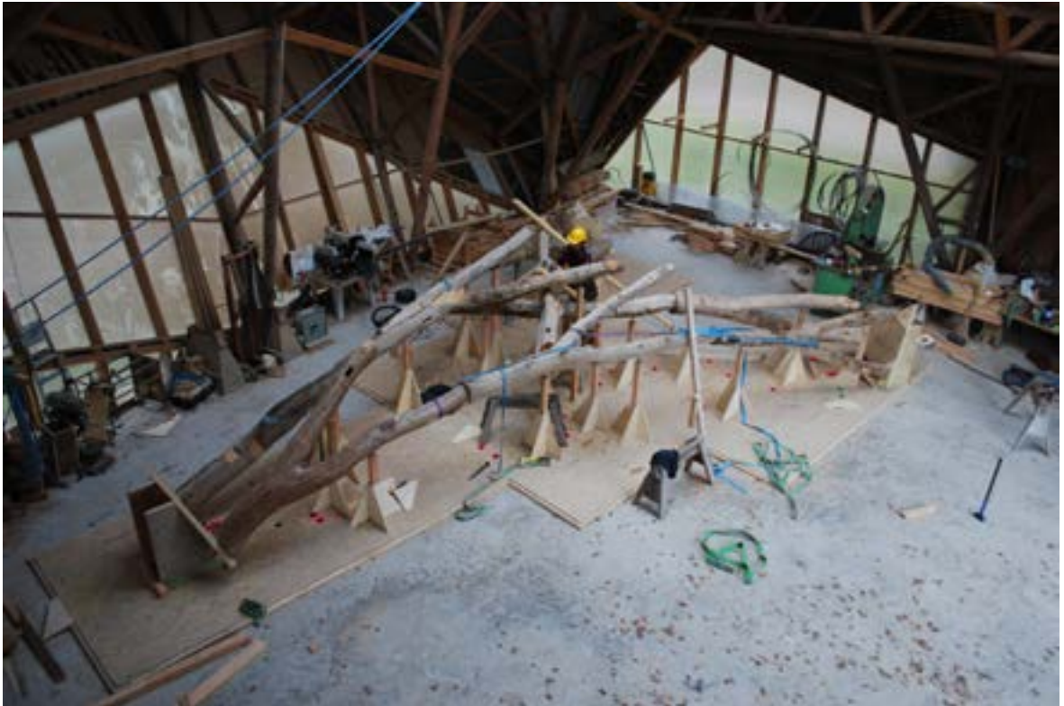
Fig. 21. The truss was pre-assembled in two halves of ten forks each. Here, the ten forks of the front half are loosely positioned together on top of the Assembly Jig before the top chords are added.
