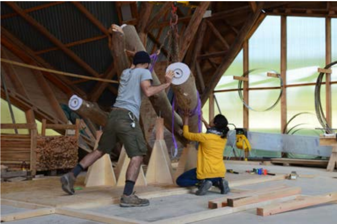
Fig. 20. Suspended in its approximate orientation, each fork was lifted in to place by the telehandler. Each was then brought to rest on their three vertical supports.
